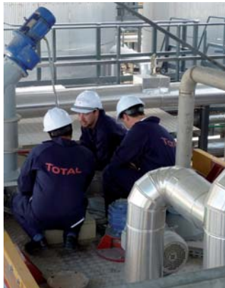
The commissioning phase was performed recently by Massenza technicians under the supervision of Total PMB specialists
